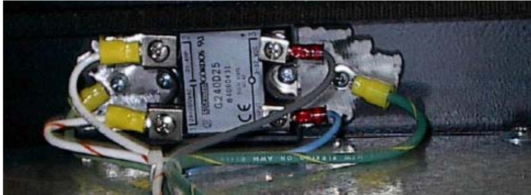
Pictured above is the solid-state relay. It is mounted beneath the diaphragm on the far right side of the access panel.
